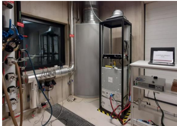
Figure 4 – PEMFC backup for system and stack characterization.
